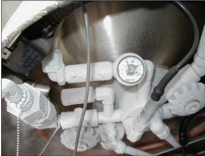
Figure 11-42m. Typical Pressure Gauge Located on the PRD Tee
