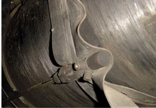
Figure 11-30d. PRD Securement Bracket and Rubber Gasket Loose
